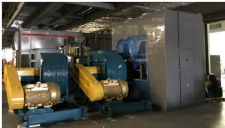
Picture 7 This Anguil LoCarb-eRCO is used in conjunction with emission concentrators to further reduce energy consumption and carbon output.
