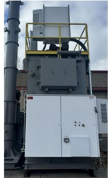
Picture 4 Electric RTOs require separate panels for heater controls
